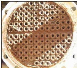
Scale inside a water-cooled chiller condenser
