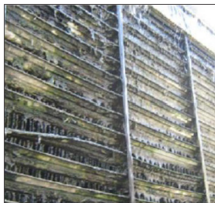
Biological growth on cooling tower inlet louvers
