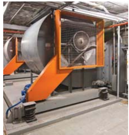
The return fans shown above are reminiscent of the supply fans that were replaced - each the size and weight of a Volkswagon Beetle.
