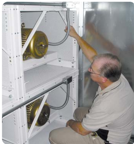
Charles Eversole, the HVAC Manager for the building, initiated the search for a fan system that would provide increased system reliability through fan-unit redundancy.
